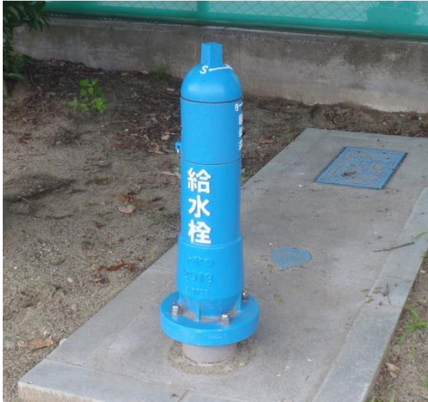
Photograph 2. Emergency water tap
